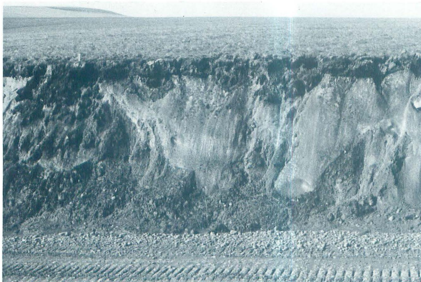
Ice masses frequently have no surface indication in natural, undisturbed terrain. This photo shows a 20-ft (6.1-m) cut slope in glacial till on the Arctic Slope about 85 mi (136.8 km) south of Prudhoe Bay.
